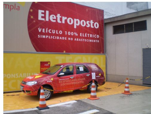
Figure 2: Recharging station at Ampla Energy Services Inc headquarter in the city of Niterói
